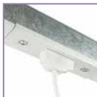
CCRT Mounted on lighting trunking
